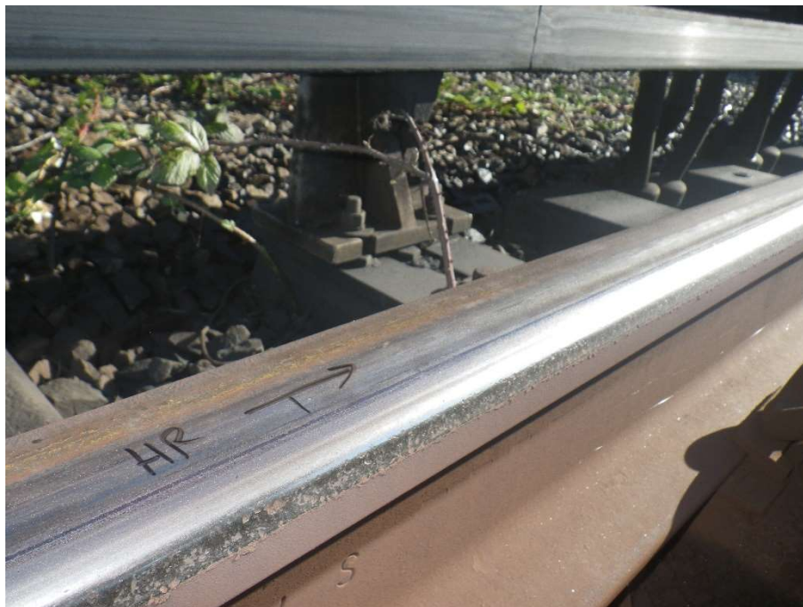
Figure 3. Gage face wear on the high rail of the test curve.
